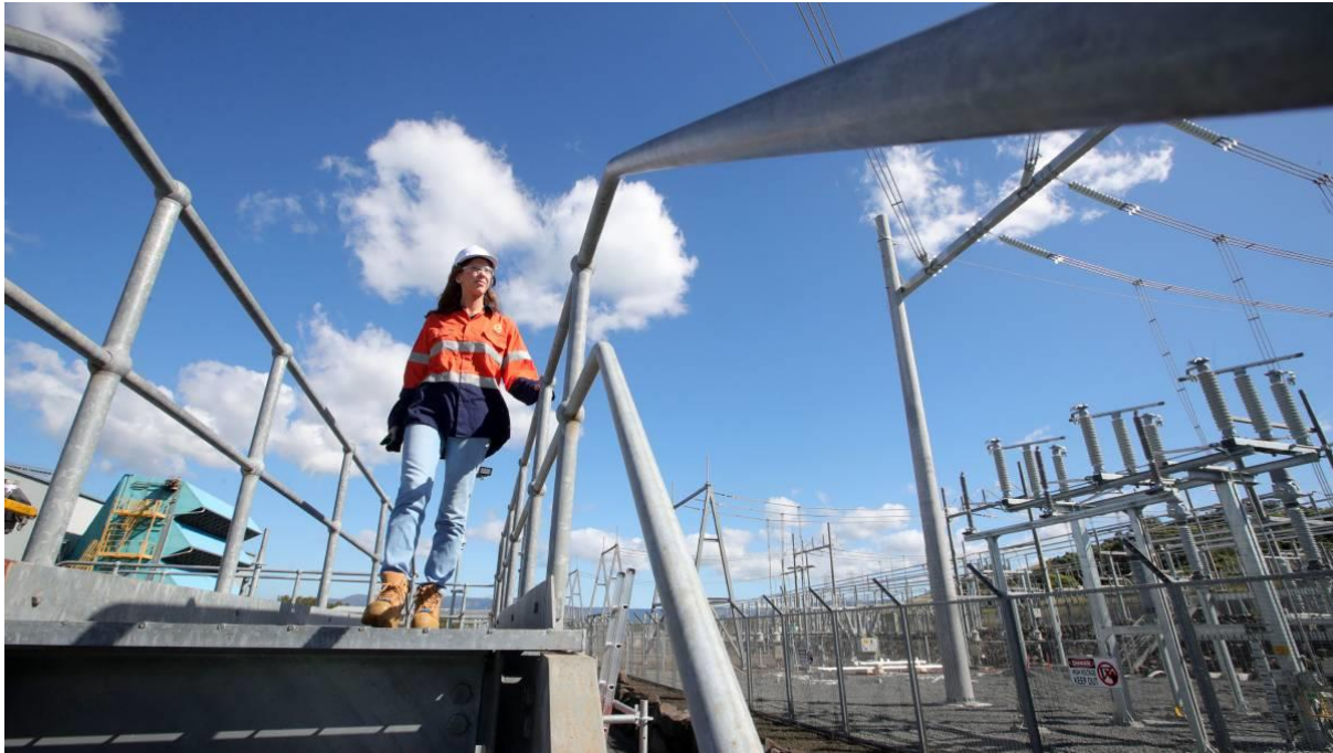
Around 300 workers are on site, including 190 local contractors, six months from completion. Picture by Sylvia Liber
