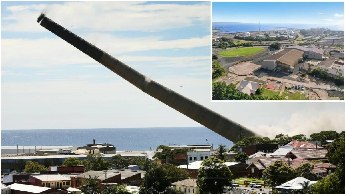
Image: The old Port Kembla copper smelter stack coming down in 2014; and, inset, the site which has been sold to a property developer. Pictures by Kirk Gilmour, Real Commercial
